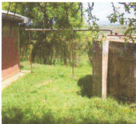
(a) Cement tank in Lembus Central
