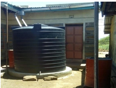
(b) Storage tank collecting rainwater in Lembus Central
